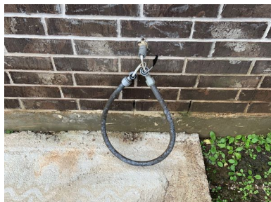
Energized electrical wires
