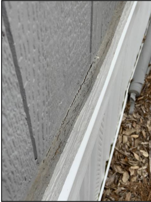
10. Caulking missing or deteriorated
