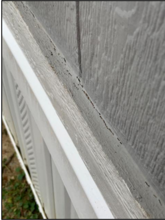
6. Caulking missing or deteriorated
