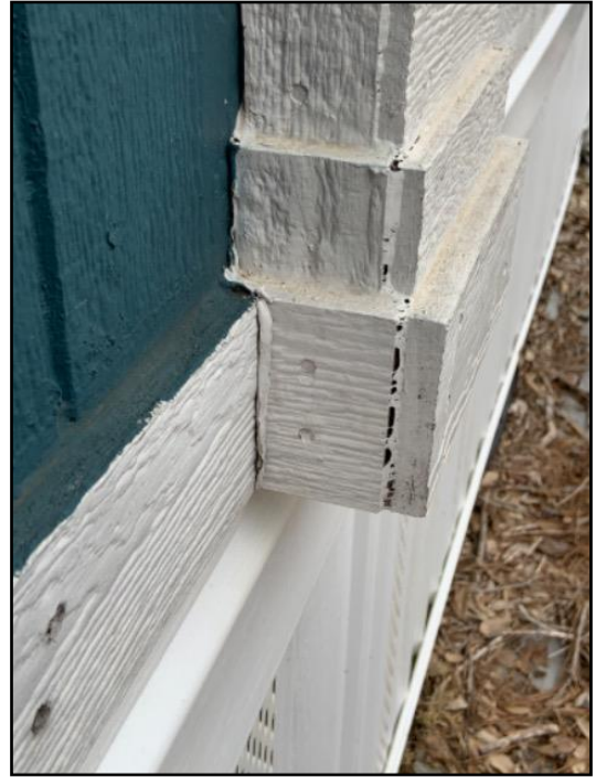
11. Caulking missing or deteriorated
