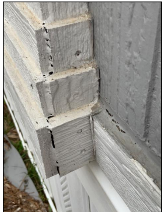
9. Caulking missing or deteriorated
