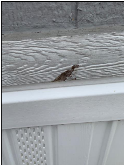
8. Caulking missing or deteriorated
