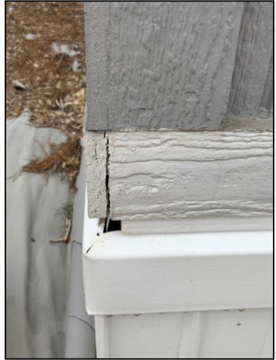
7. Caulking missing or deteriorated
