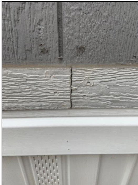
12. Caulking missing or deteriorated
