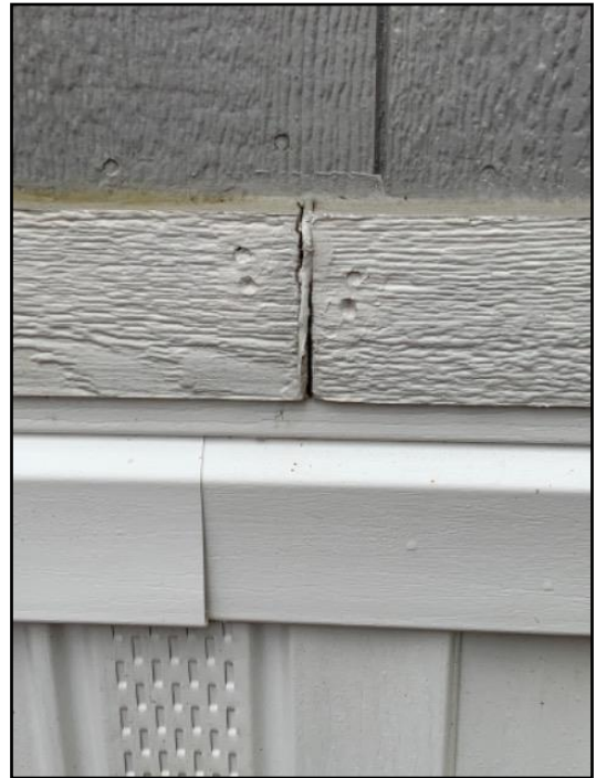
5. Caulking missing or deteriorated
