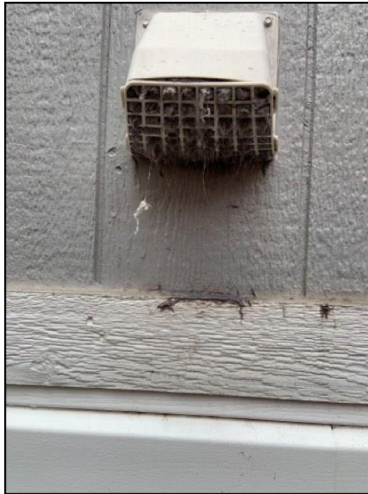
17. Dryer vent obstructed
