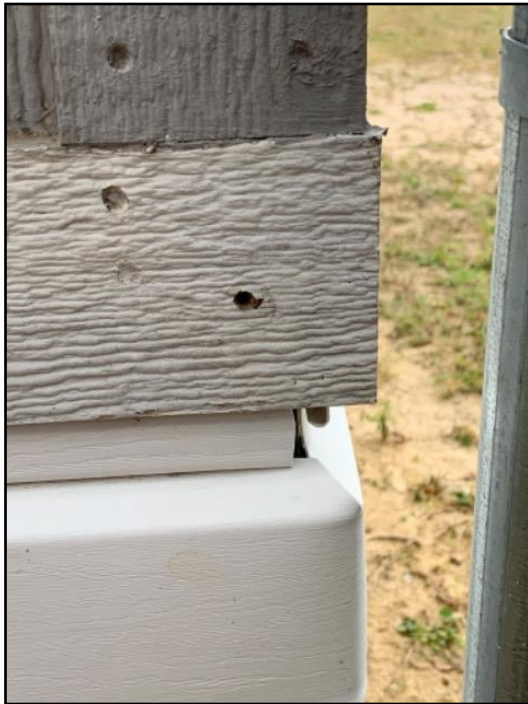
4. Caulking missing or deteriorated
